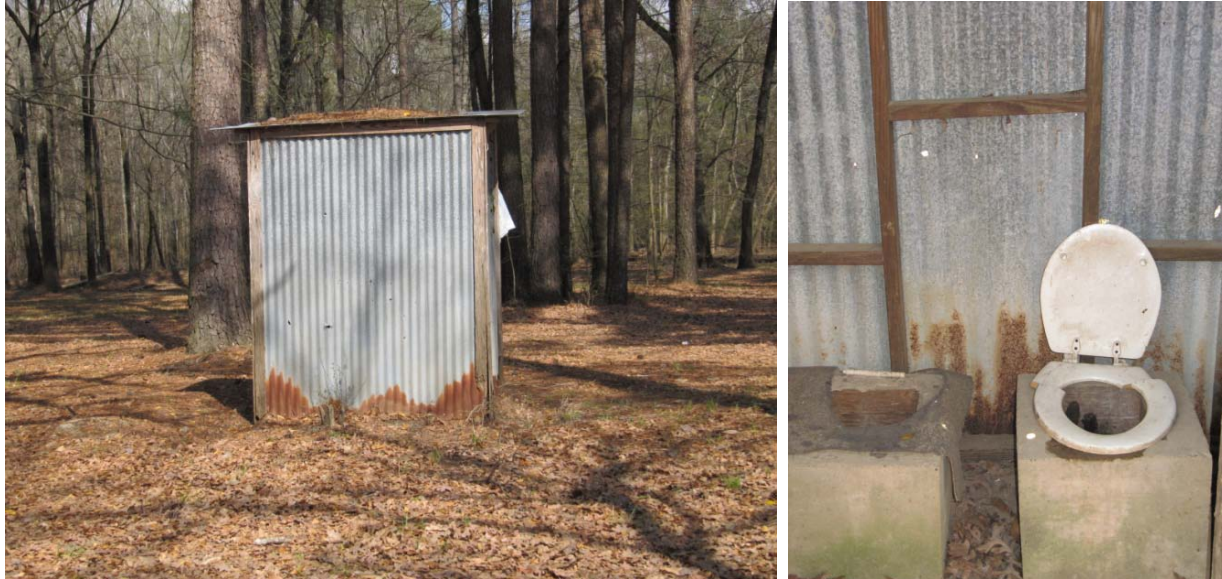
Figure 4. Yellow Dog-Site 1: Pit toilet building; Interior needs maintenance
